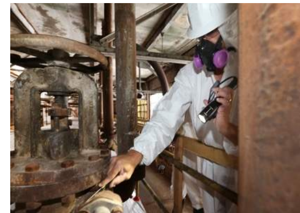
ASBESTOS CONTAINMENT AREAS
